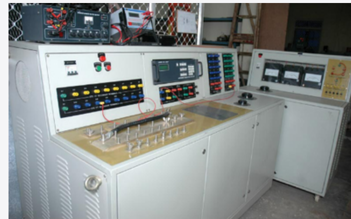
High Voltage Test
